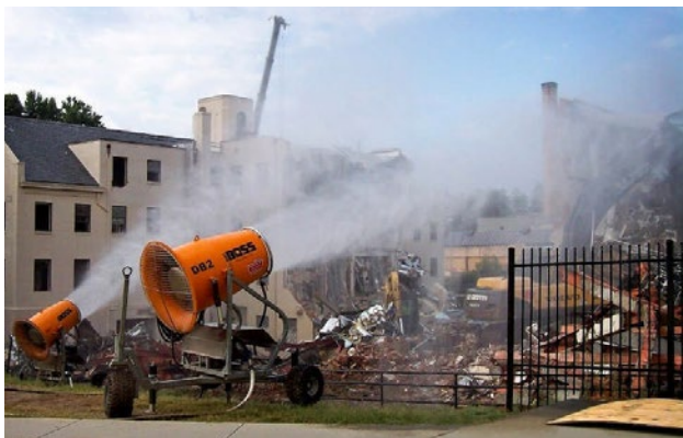
Atomized misting canons, like the DustBoss unit pictured, are an effective way to suppress silica dust.
